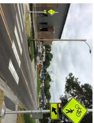
Rectangular rapid flashing beacons are activated by pedestrian push buttons.
