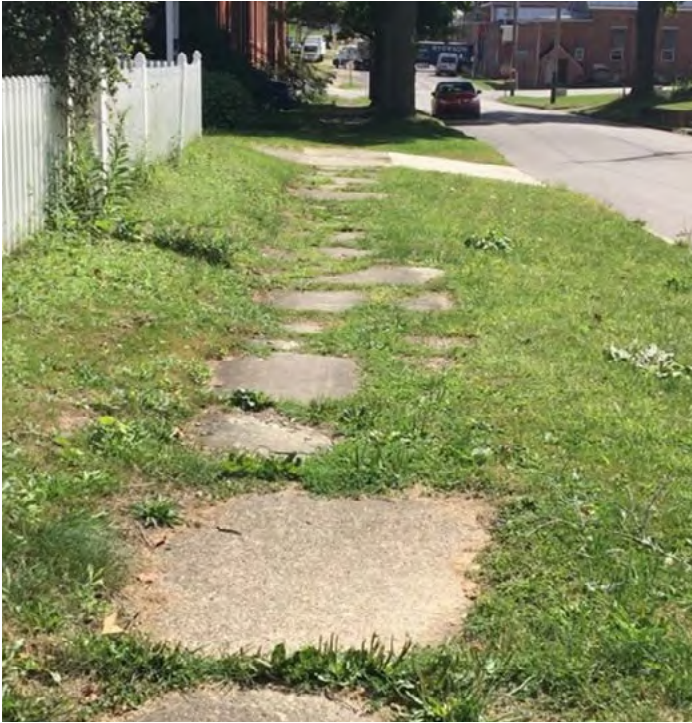
Some concrete sidewalks have deteriorated to the point that cracking, heaving, or settling have made them very uneven.
